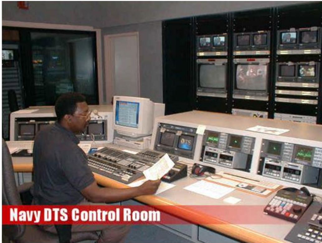
Figure 5-3 — Navy DTS Control Room.
